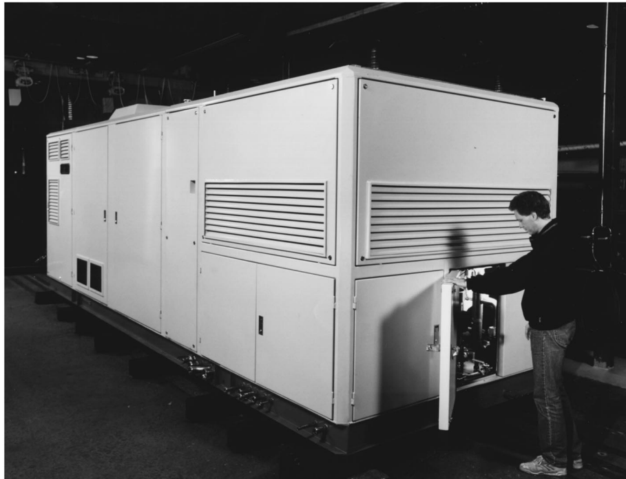
Fig. 1. Prototype natural gas fueled PEM power plant.
