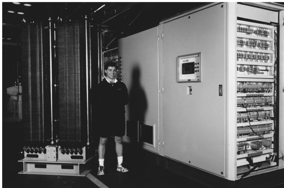
Fig. 2. Stationary PEM fuel cell.
